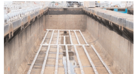
Newly installed fine pore diffusers significantly lower energy costs.
